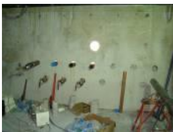
Piping array entering building
