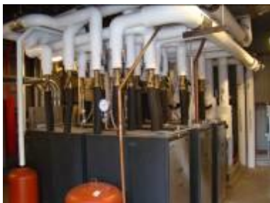
Water to water heat pumps
